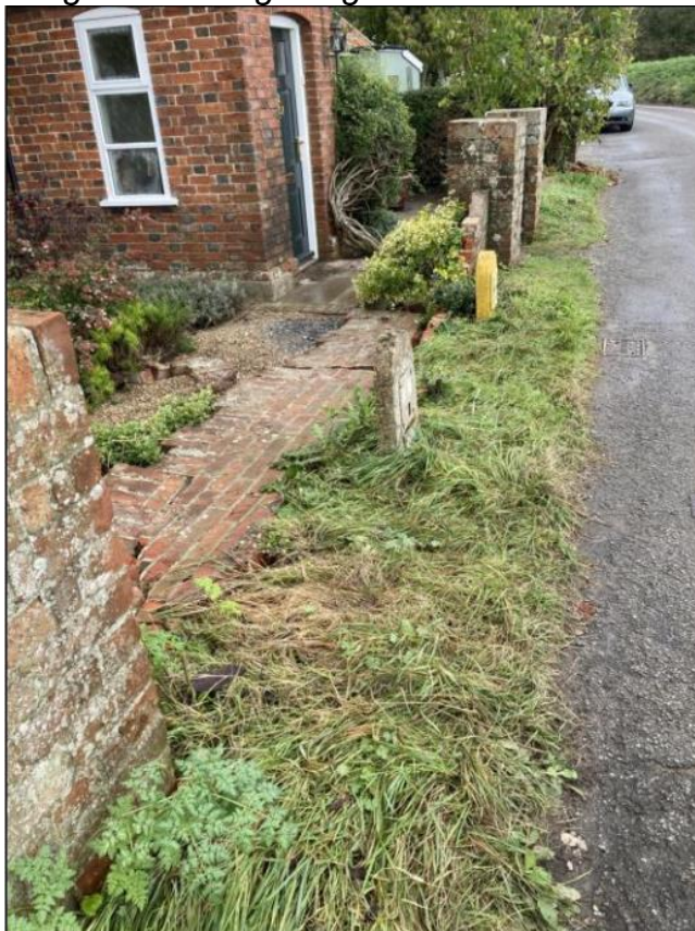
Image 7 - Damage to garden wall on Fairfield Road
